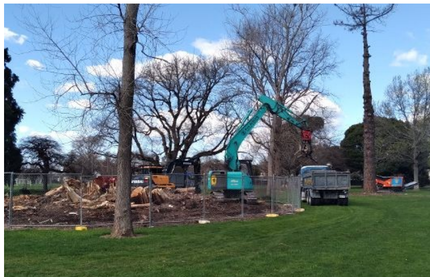
Nearly all gone, except for the massive above-ground root pad.
